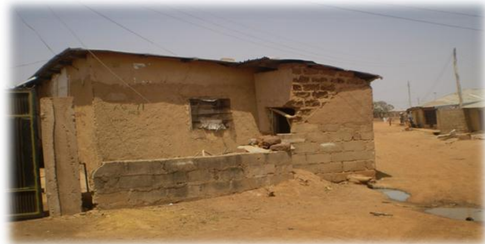
Fig. 2: Sewage disposal from houses into the streets Source: Authors Fieldwork, 2012
